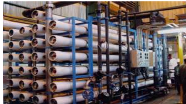
Reverse osmosis desalination **
