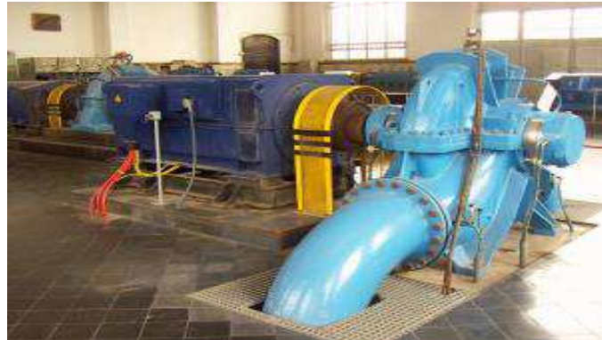
Raw water intake **
