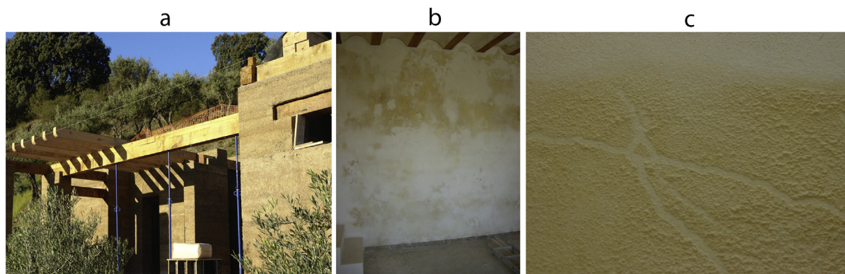
Fig. 1. (a) A house built with rammed hemp concrete walls; (b) pathologies arisen on the plaster of a hemp concrete wall on the inner Northern side of a hemp concrete building (c) detail of the powdered aspect of the yellowish deposition on the same plaster. (For interpretation of the references to colour in this figure legend, the reader is referred to the web version of this article.)
