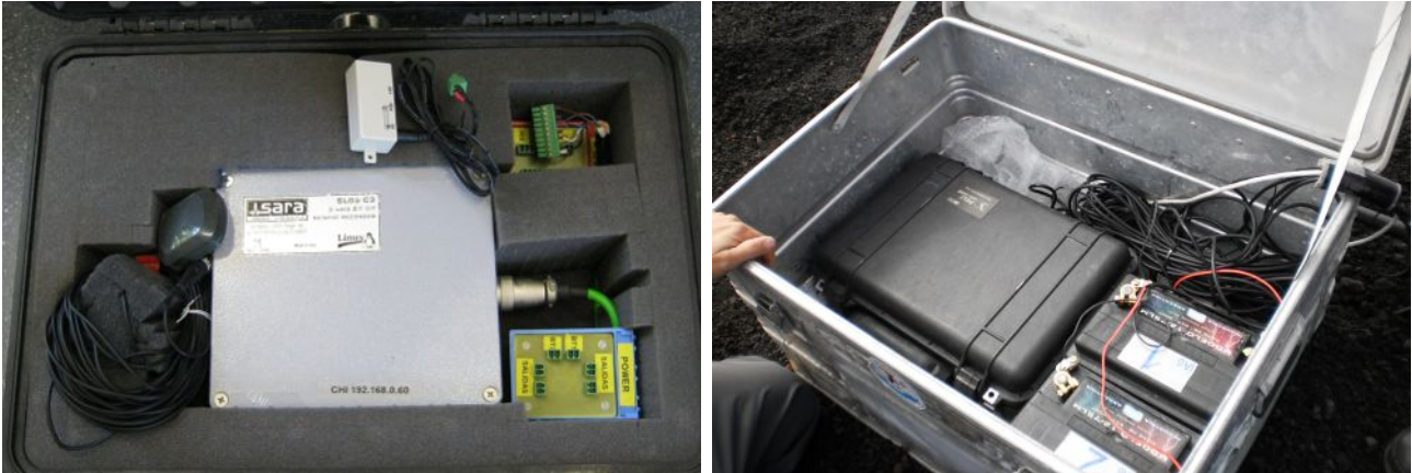
Figure 4. Left: SARA data acquisition system embedded in a waterproof PELI case; right: SARA data acquisition system and two batteries in an aluminum box for further protection.
