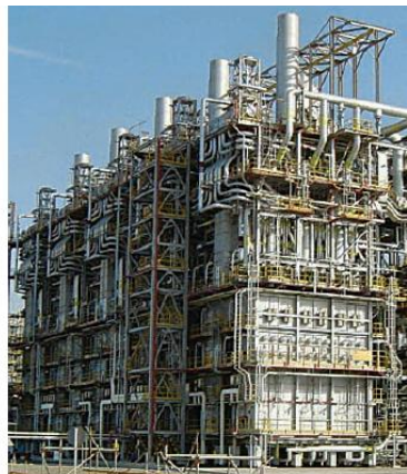
Figure 5. Furnace section of a modern ethylene plant
